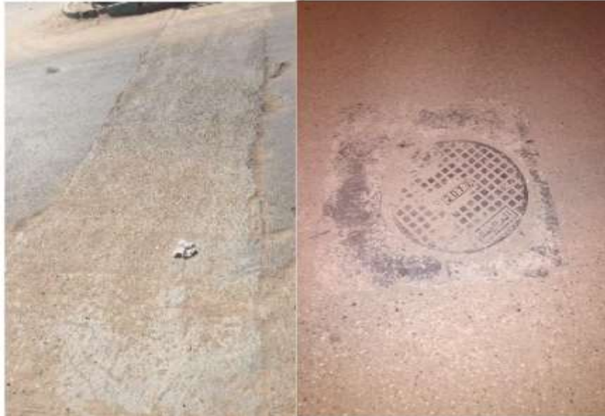
Figure 14 Patching and utility cuts in study area
