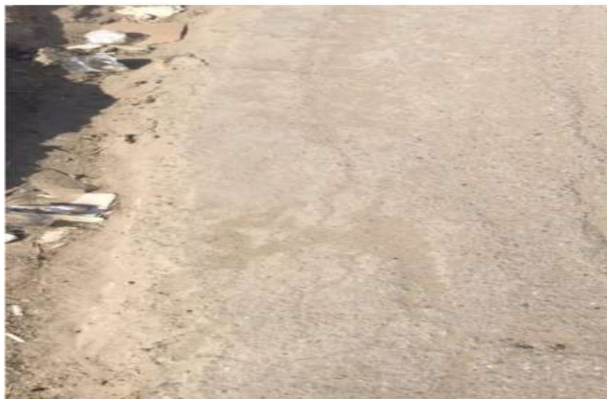
Figure 8 Edge crack in study area
