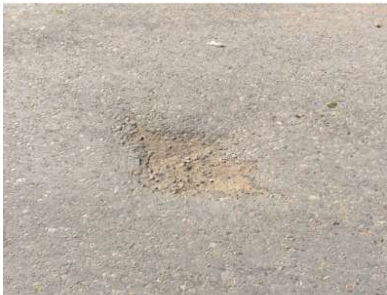
Figure 11 Pothole in study area
