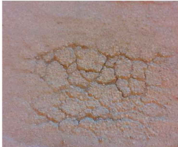
Figure 7 Alligator cracks in study area
